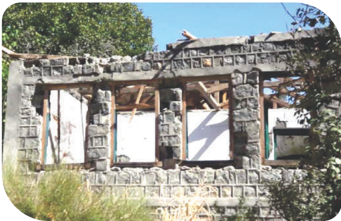
Chitral – Damaged School
